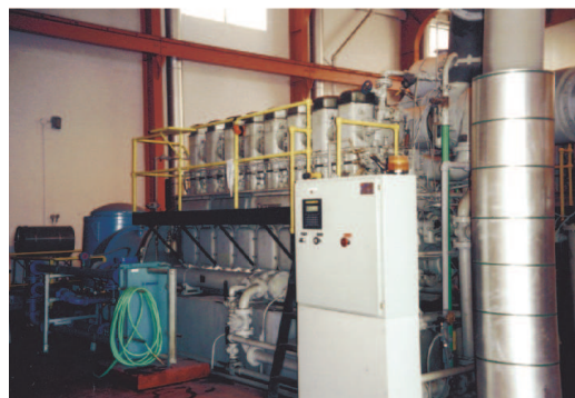
Figure 7-4. Diesel Engine of Pump Station
