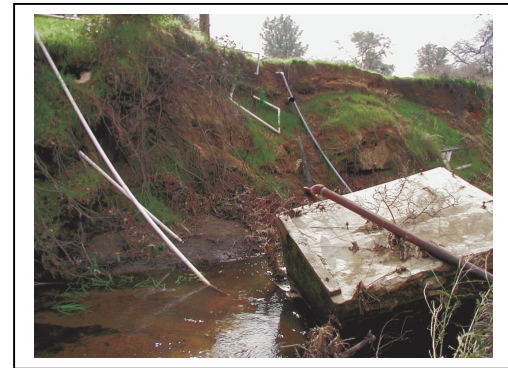
PUMPS, PIPES AND GARBAGE NEAR PENRYN ROAD (PHOTO COURTESY B. WASHBURN)
