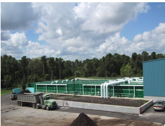
Figure 7-5: The Wright Environmental in-vessel system.
