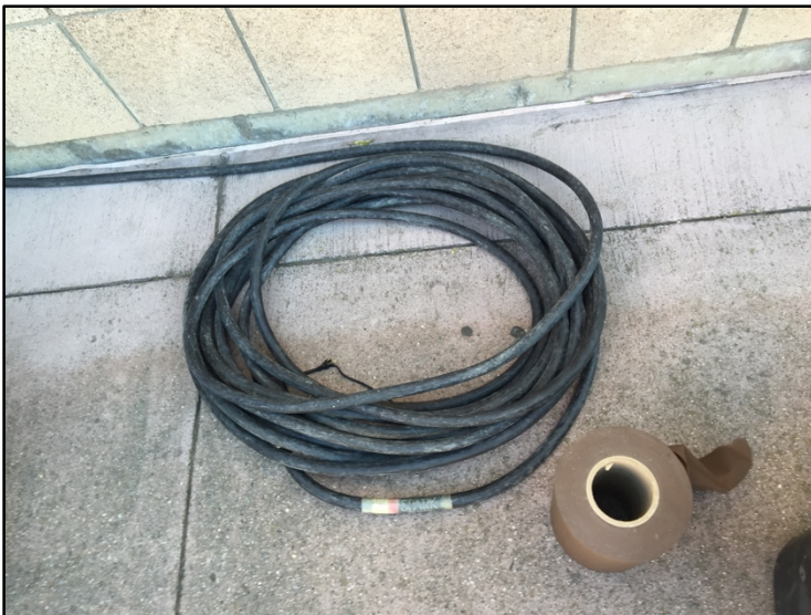
Figure 5 Example of heavy cabling used for event lighting
