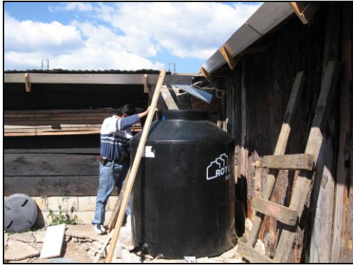
Figure 4. Implementing a domestic rainwater harvesting system in Cinco de Marzo
