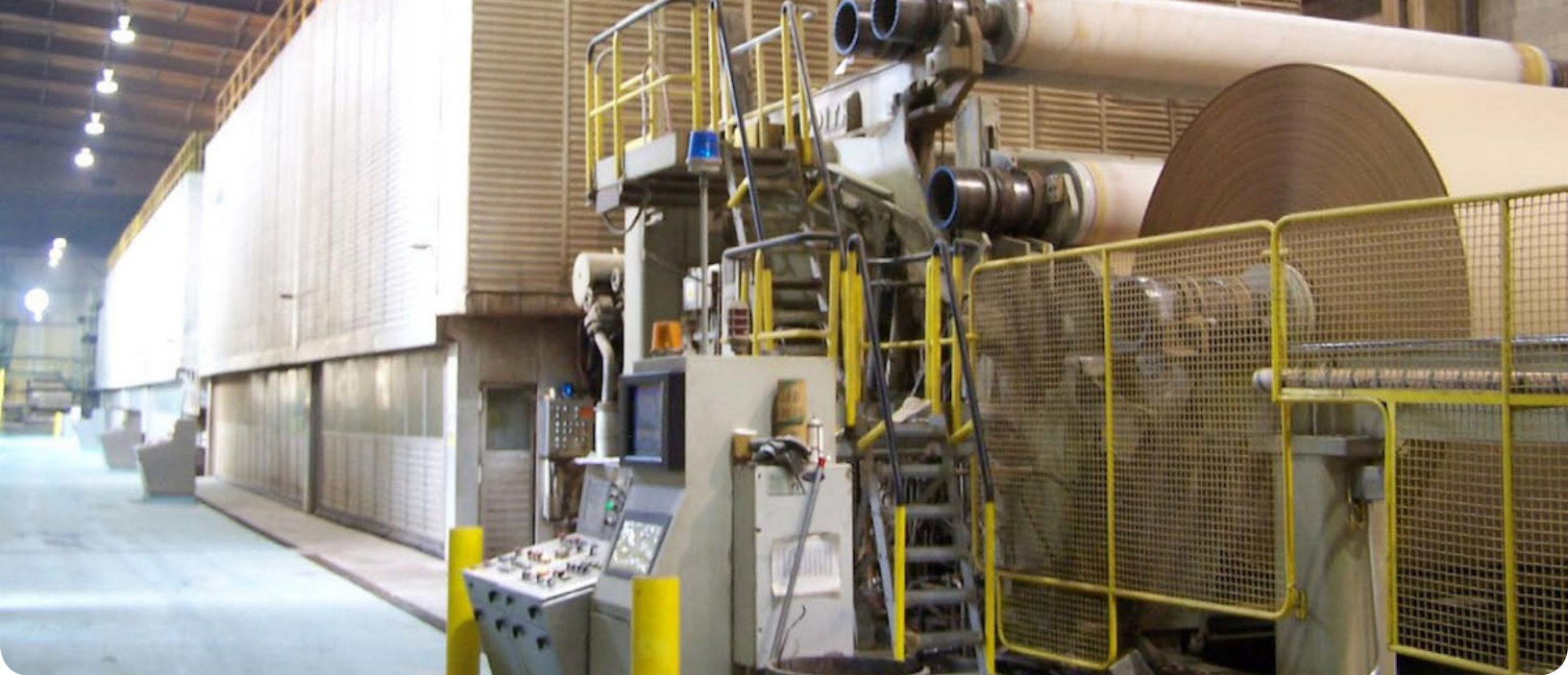
Paper production facility. Source: Pratt Industries
