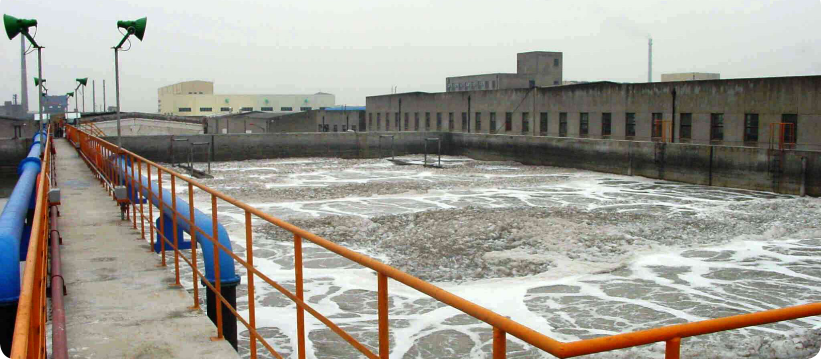
Paper production facility wastewater treatment. Source: ADI Systems
