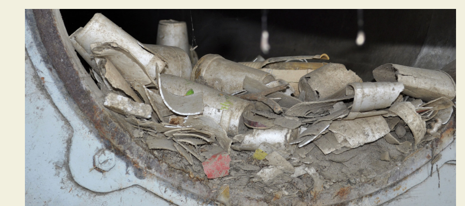
San Gabriel River Storm Drain (Photo: Michael Mori)
