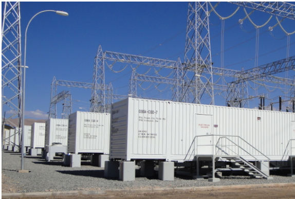
Figure 2.3 - A123 Systems 12MW battery in Chile. (Source: A123 Systems, 2011)
