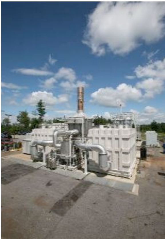
Figure 2.13 - 2.8 MW fuel cell power plant designated ultra clean by CARB (Source: FuelCell, 2012)
