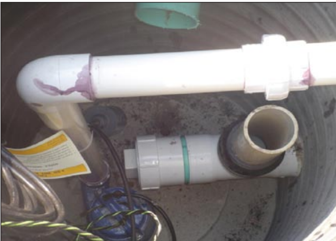
Figure 6b. Sump basin station showing pump, water level adjustment, and quick disconnect to service the pump.
