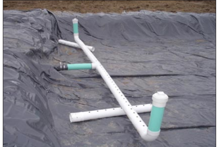
Figure 4. Collection 4" PVC manifold at the outlet end of the wetland.
