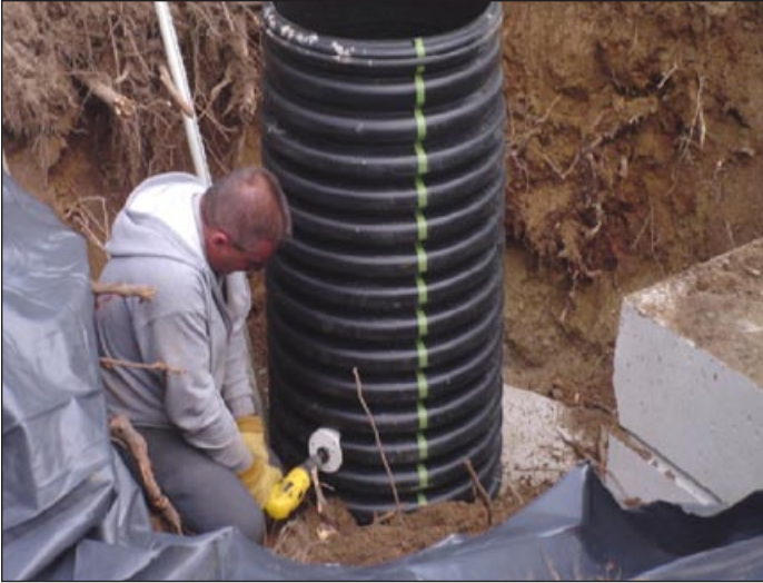
Figure 6a. Sump basin station using 24" drain tile.
