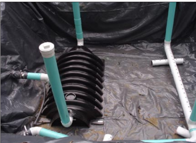
Figure 3. Wetland cell using a plastic chamber as an inlet-end manifold and 4" PVC pipe as an outlet-end manifold with clean-outs.
