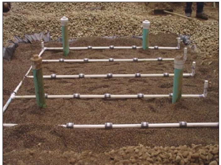
Figure 8. Recirculating 1" PVC manifold, pressure laterals, and orifice shields.
