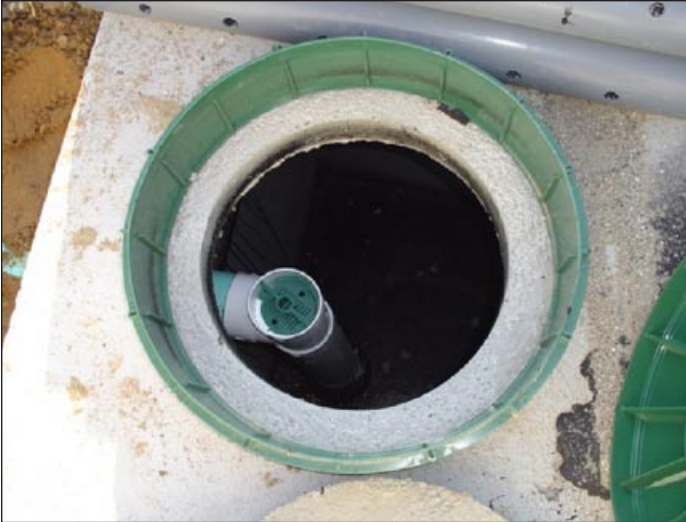
Figure 2. Effluent filter in place at the septic tank outlet.
