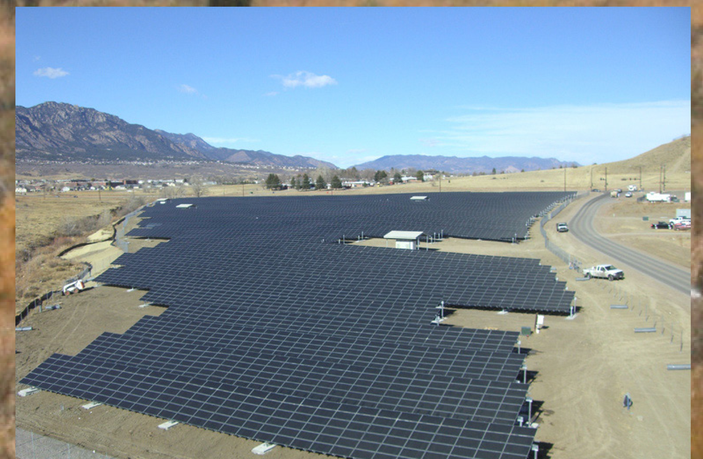
Fort Carson PV array on site previously used as landfill (photo: US EPA Repower America)
