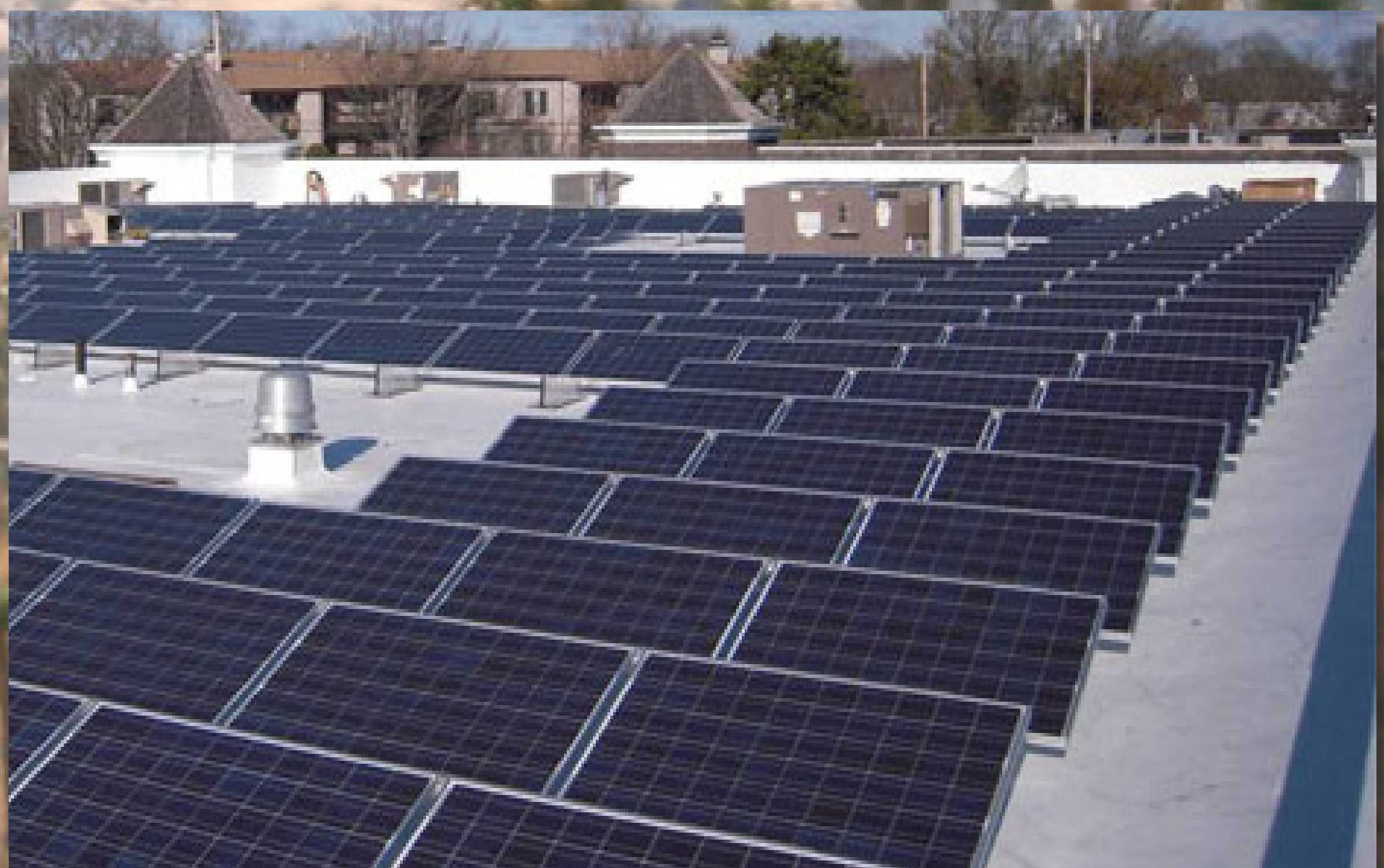
Commercial and apartment rooftops are well suited to community solar applications
