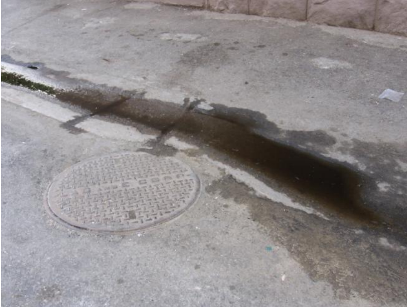
Water collecting in the middle of the alley due to sloping towards the center
