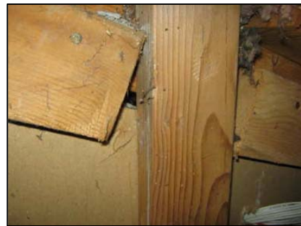
Image 1: Hole allows air to flow in and out between living room and garage.
