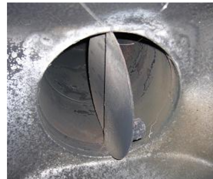
Image 2. Fireplace damper should be closed when not in use.
