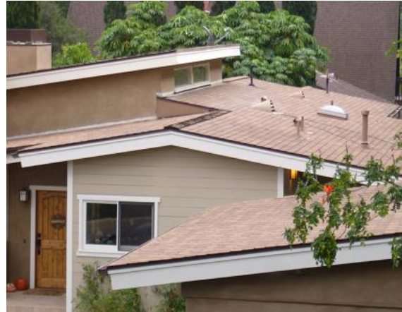
Image 1. Additional weather-stripping may reduce air leakage.
