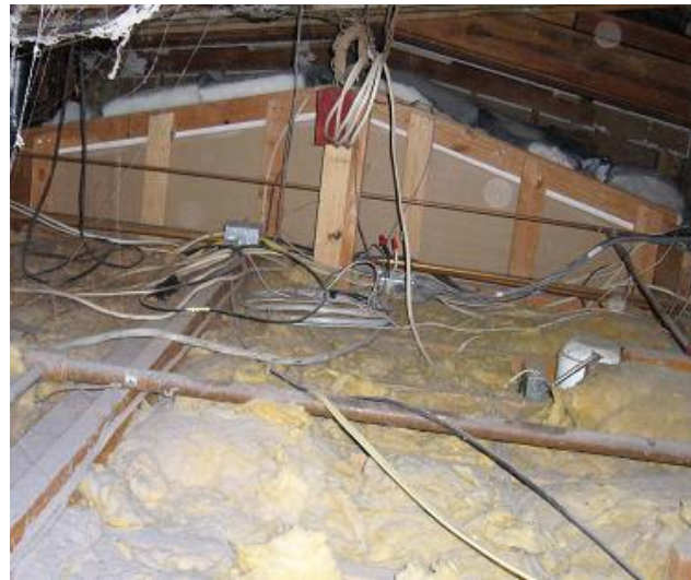
Image 3. Existing attic insulation shows old age and discoloring. Much of it is missing.
