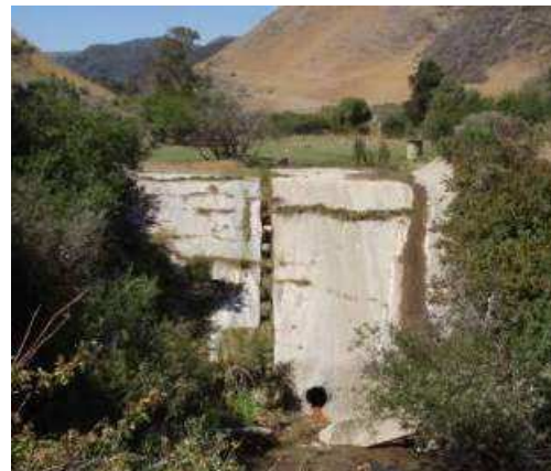
Figure 4. The Santa Anita Creek Dam.
